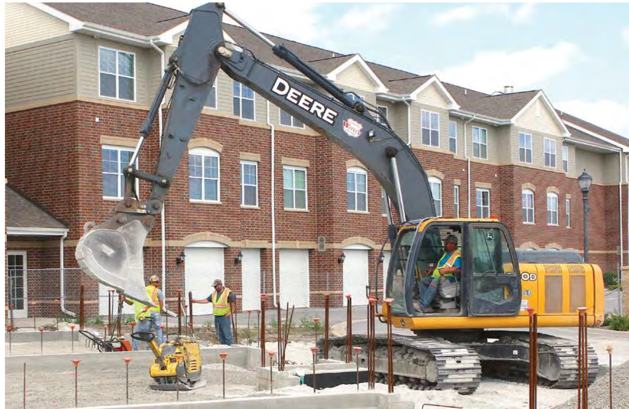
With initial planning and groundbreaking completed, construction is well underway for Phase II of Park Place of St. John retirement living apartments, which will allow more than 50 new residents to move in.
